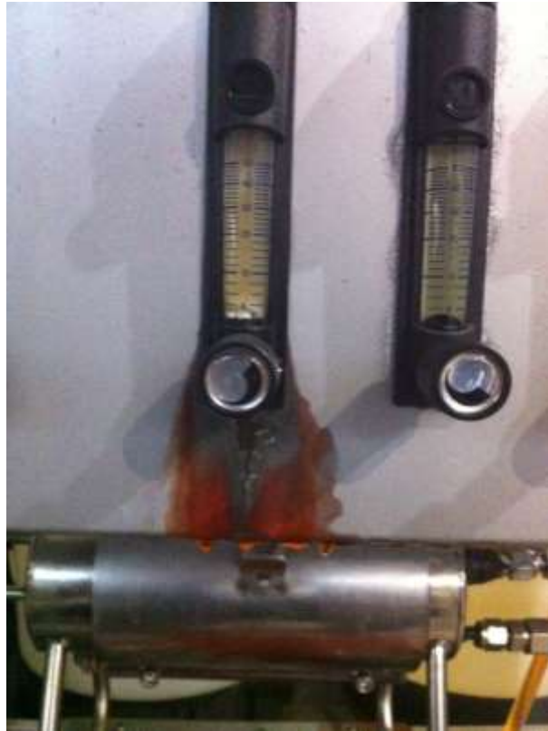
Figure 14: Flow meter that was corroded by the absolute ethanol which contained KOH
