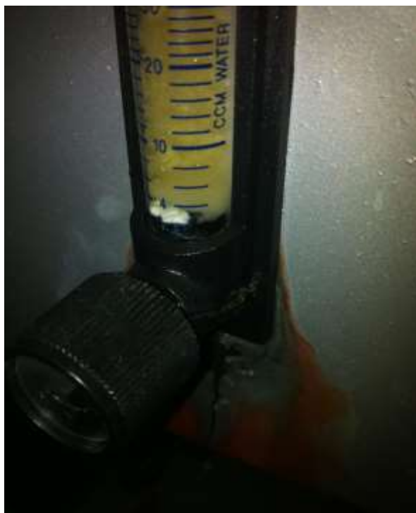
Figure 13: Flow meter that was broken caused by the over pressure created by the pump due to the fatty acid stuck in it.
