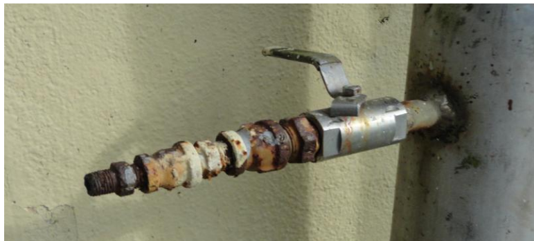
Figure 3.4 (b): Fitting connected of Pilot Plant Seriting Hilir
